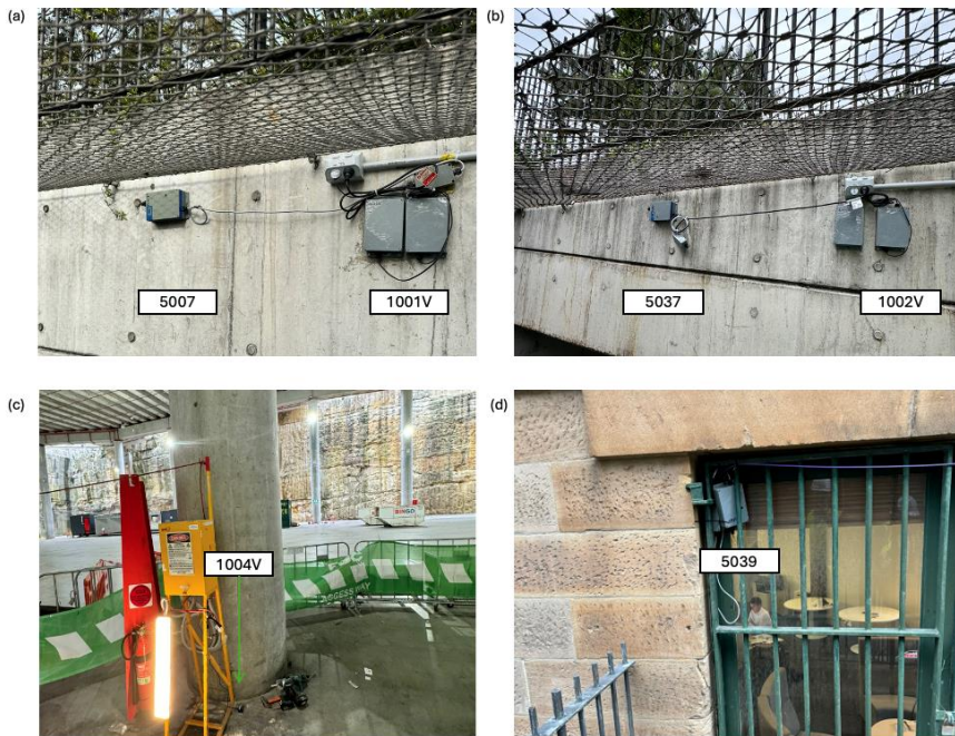
Figure 3: Shows the installed sensors on the Cutaway project site: (a) 5007 & 1001V, (b) 5037 & 1002V, (c) 1004V, and (d) 5039.
