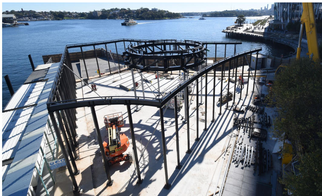
Progress to date: erecting structural steel for columns and preparing the oculus for installation
