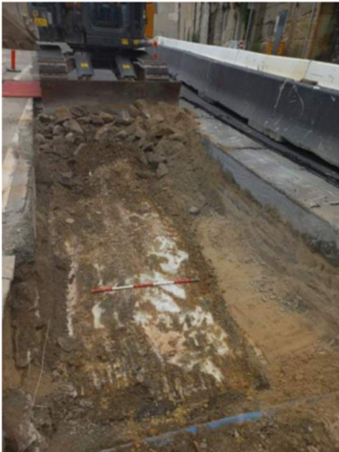
Figure 4.12: Cut bedrock observed in the base of Trench 2.2. The High Street wall is visible in the background. AMBS 2024, Figure 4.17.
