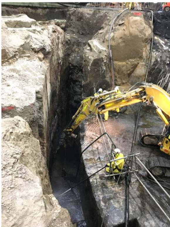
Figure 4.24: Excavation of the 1882 gasholder, excavated into the natural sandstone, under Hickson Road. Lendlease 2019.
