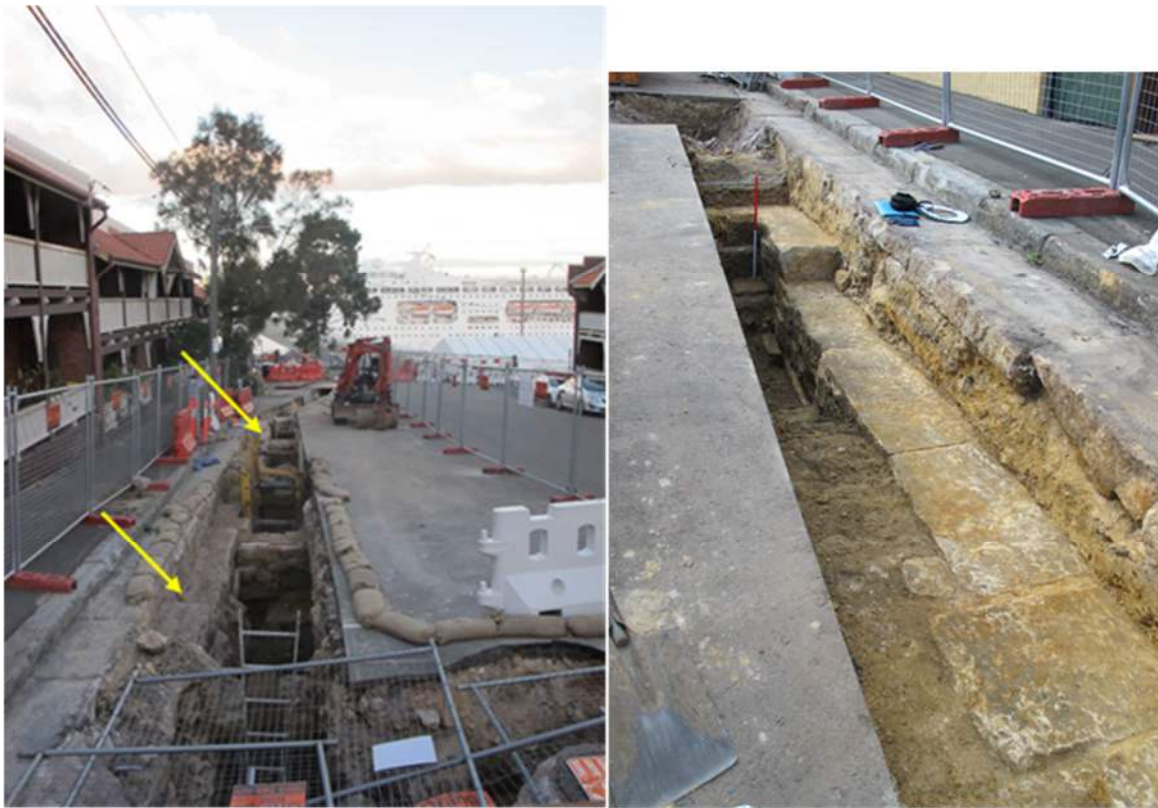
Figure 4.14: Trench for new stormwater service on the southern side of High Street. Left: The arrows indicate the main southern wall of the building which extended deep below the current street level. Right: View to east showing detail of the main sandstone wall.
