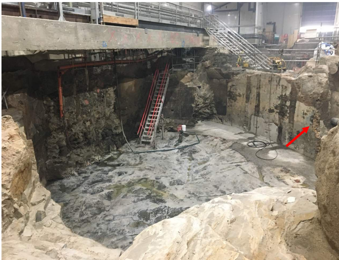
Figure 4.29: Excavation of the small gasholder under Hickson Road, cut into bedrock. A section of brick wall is visible to one side (arrowed). Lendlease 2019.
