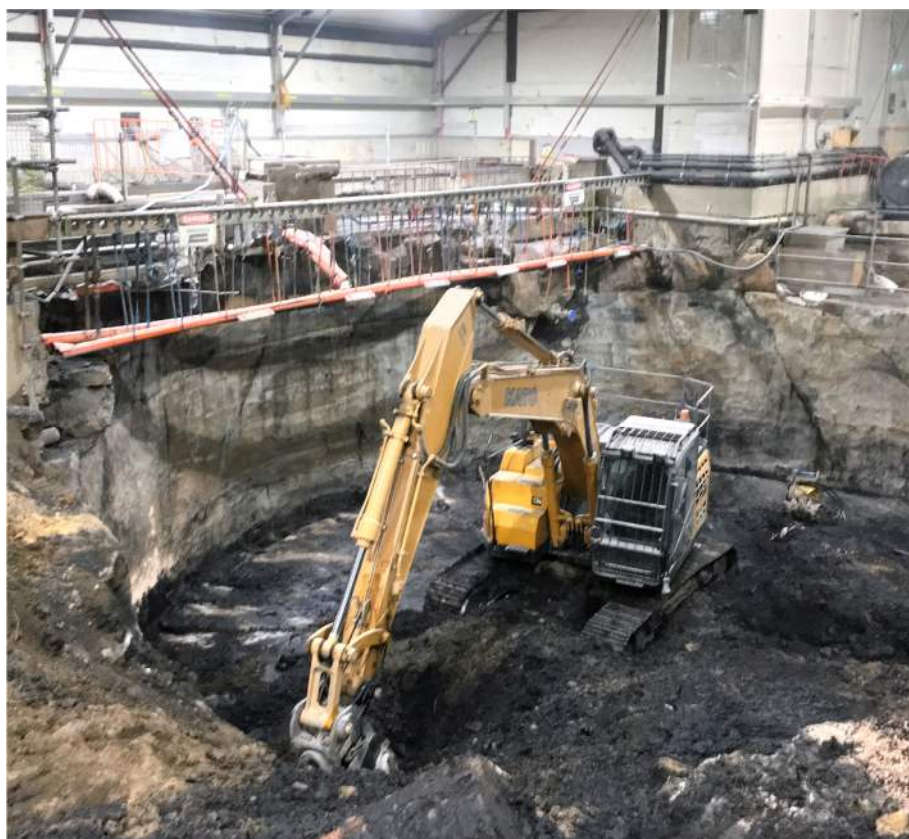
Figure 4.26: Cleaning out of the tar tank, excavated into the natural sandstone, under Hickson Road, cutting sandstone bedrock. Lendlease 2019.
