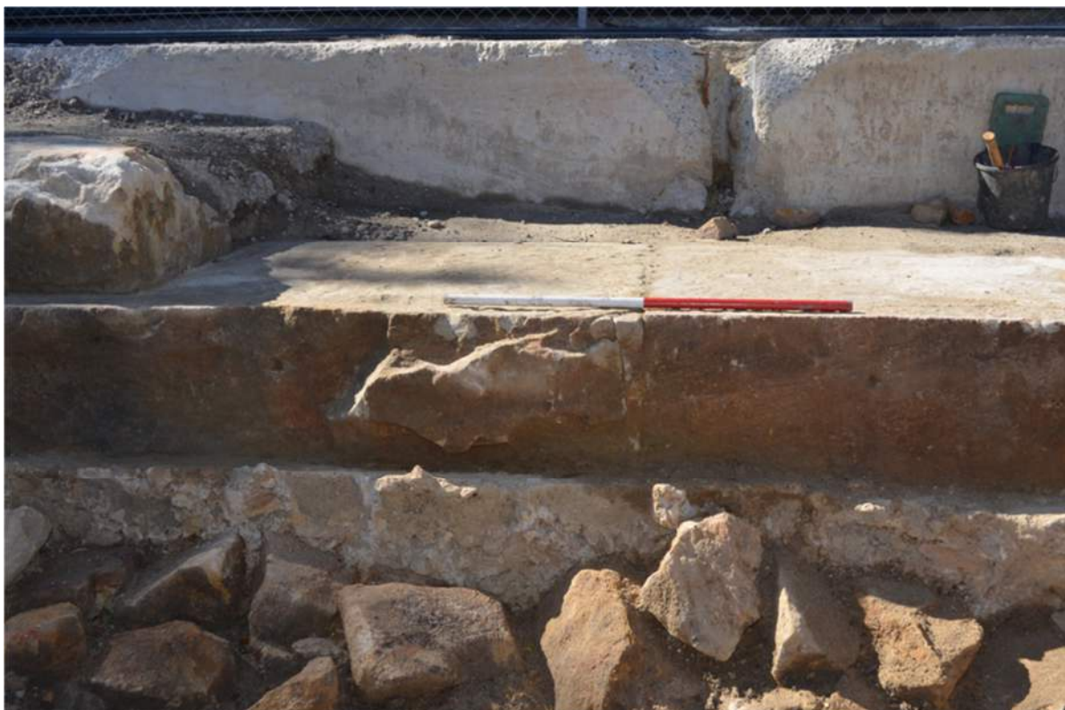
Figure 4.5: The footing of the Grafton Bond Store showing the sandstone rubble 'formwork' (bottom), the cyclopean concrete (context 12813 above), and the lowest course of sandstone blocks (centre of image, context 12806). Scale 1m. View to east. Casey & Lowe 2022d.
