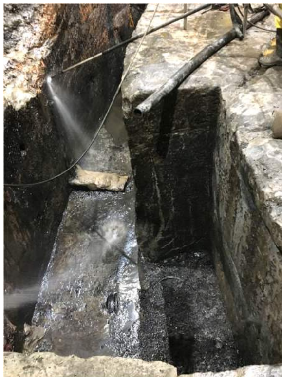
Figure 4.25: Excavation of the 1882 gasholder, excavated into the natural sandstone, under Hickson Road. Lendlease 2019.
