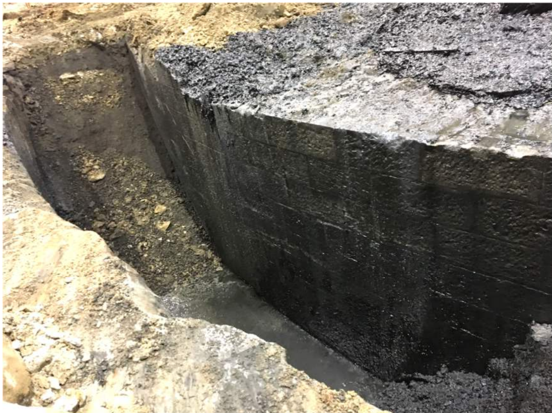
Figure 4.21: Excavation of the 1870s gasholder annulus within Block 4, showing the worked sandstone blocks used in the construction. Lendlease 2019.
