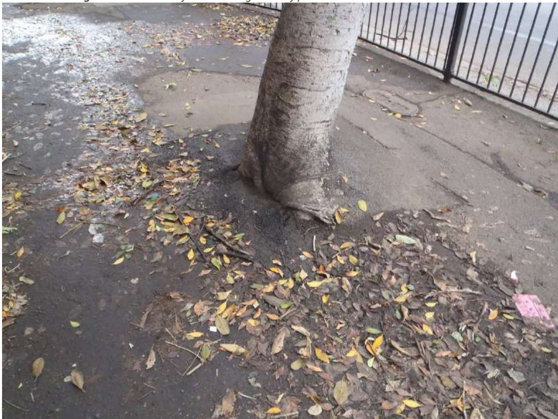
Figure 26. The base of T13 Hill's Fig. Date of photo: 28 October 2025. Source: ELKE
